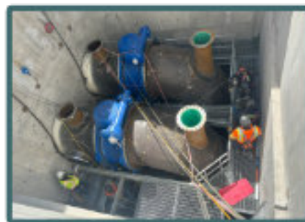
Grating and handrails at Landing 2 around the new 72-inch butterfly valves and bypass piping
